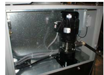
Machine Feed Pump
