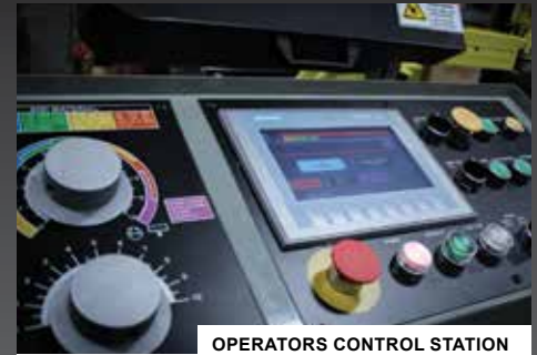
OPERATORS CONTROL STATION
