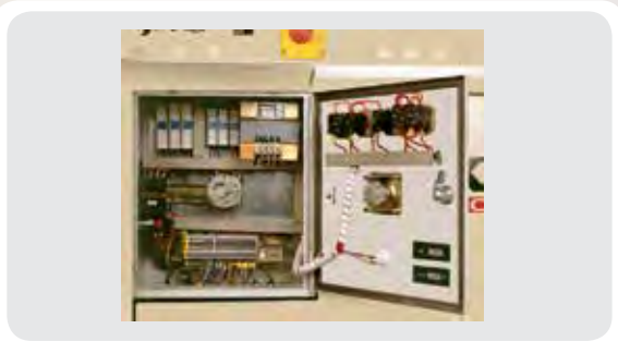
Electrical box with safety and integrated controls
