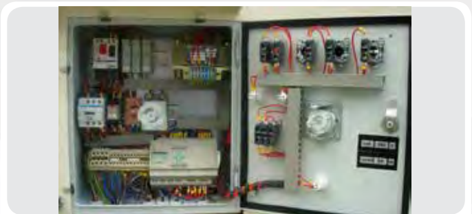
Electric panel with overload protection elements and integrated controls
