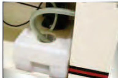
Coolant System Reservoir
