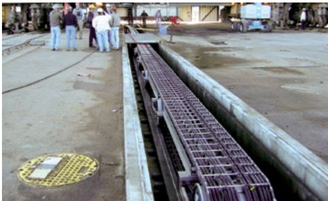
Custom stainless steel Gortrac® LRC carrier system with rolling carriage for a rocket launch system in California. Driven end modified for customer's application requirements.
