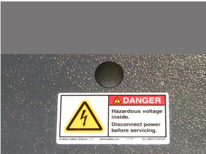
Located on the cover of the main electrical panel.
