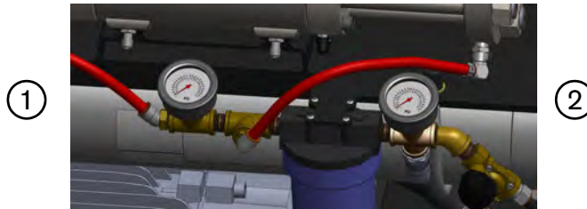
1 Postfilter water-pressure gauge
