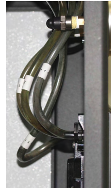
Bad tube routing
